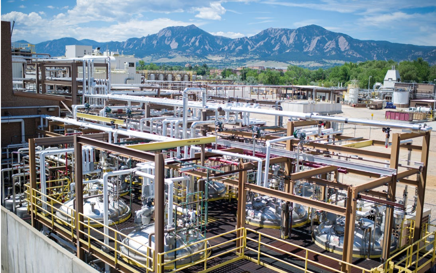
CordenPharma Colorado (USA) utilizes more than ten 50m 3 tanks to support our green manufacturing concept.
